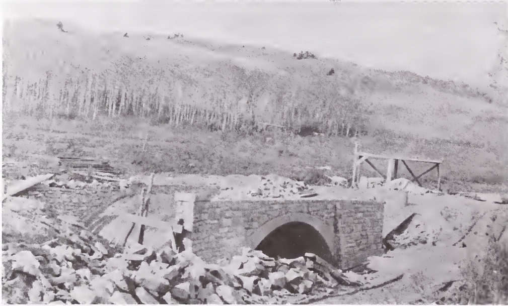
The Kiowa Bridge. Built by Evarts Blakeslee in 1928, the photograph shows the bridge prior to the construction of the deck (photograph courtesy of Robert Blakeslee).
